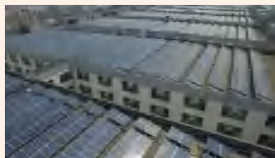
Factory roof solar photovoltaic panels
